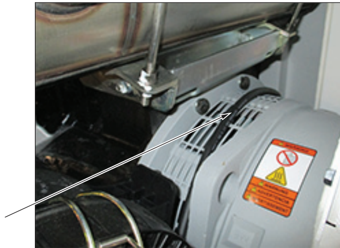
Figure 15 - Harness Routed Over Generator
