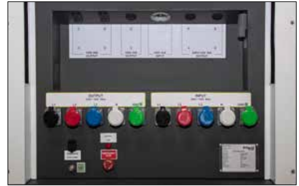
Shown here is 3-phase input/output for the MBE30
